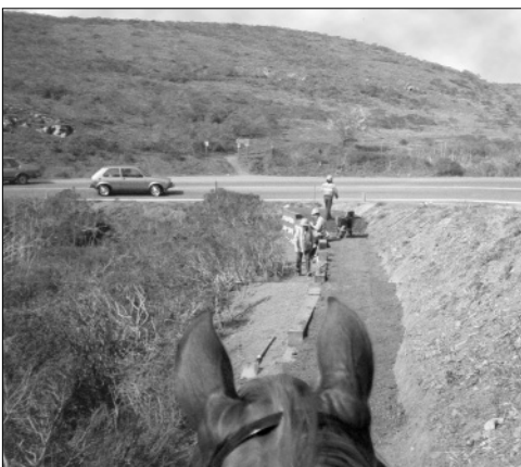
Marin Conservation Corp constructs multiuse segment of Bay Area Ridge Trail so riders can avoid riding on congested Hwy One above Muir Beach.
